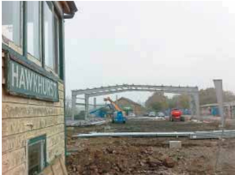
MODERN TWIST: Hawhurst Station Business Park is incorporating parts of the former railway site
